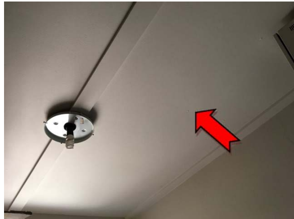
Photo 4. Interior, ground level, eastern elevation, toilet 2, ceiling – asbestos-containing fibre cement sheeting.
