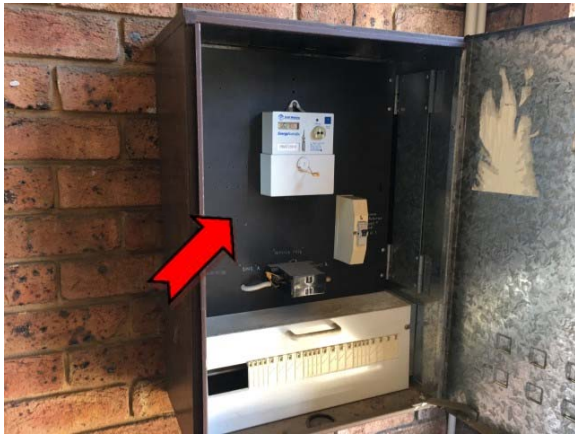
Photo 3. Exterior, ground level, western elevation, switchboard – suspected asbestos-containing bituminous backing board.
