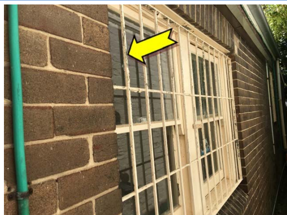
Photo 6. Exterior, ground level, throughout, window frames – lead-containing beige upper coloured paint system.
