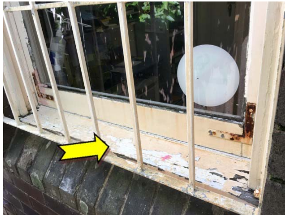
Photo 7. Exterior, ground level, throughout, window frames – lead-containing white lower coloured paint system.
