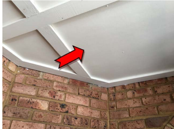
Photo 2. Exterior, ground level, entrance lobby, ceiling – asbestos-containing fibre cement sheeting.
