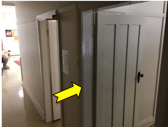
Photo 9. Interior, ground level, throughout, doors and door frames – suspected lead-containing white upper coloured paint system.
