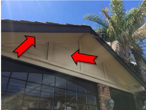
Photo 1. Exterior, ground level, western elevation, eaves and gable – suspected asbestos-containing fibre cement sheeting.
