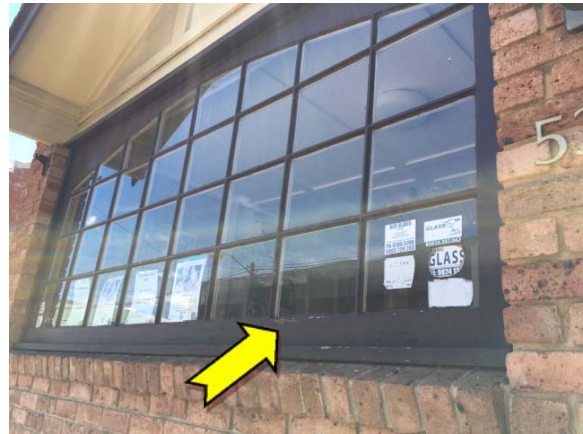
Photo 8. Exterior, ground level, throughout, window frames – suspected lead-containing brown upper coloured paint system.
